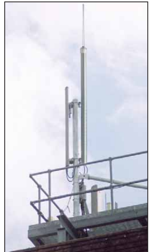
Illustrators representation of installed ERITECH Isolated Downconductor system
